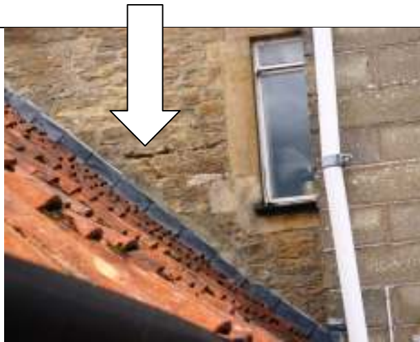
Weathered joint on rear wall
